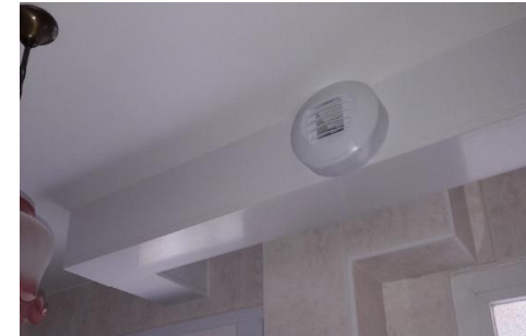
Soffites de raccordement VMC
