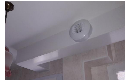
Soffites de raccordement VMC
